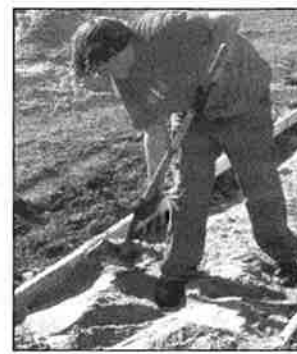
LEVELING SAND, junior Rob Merry works on the new sidewalk after school Oct. 7. The walk, made by the ag class, was added to the west side of the school. PHOTO BY JESSICA AUGUSTINE
